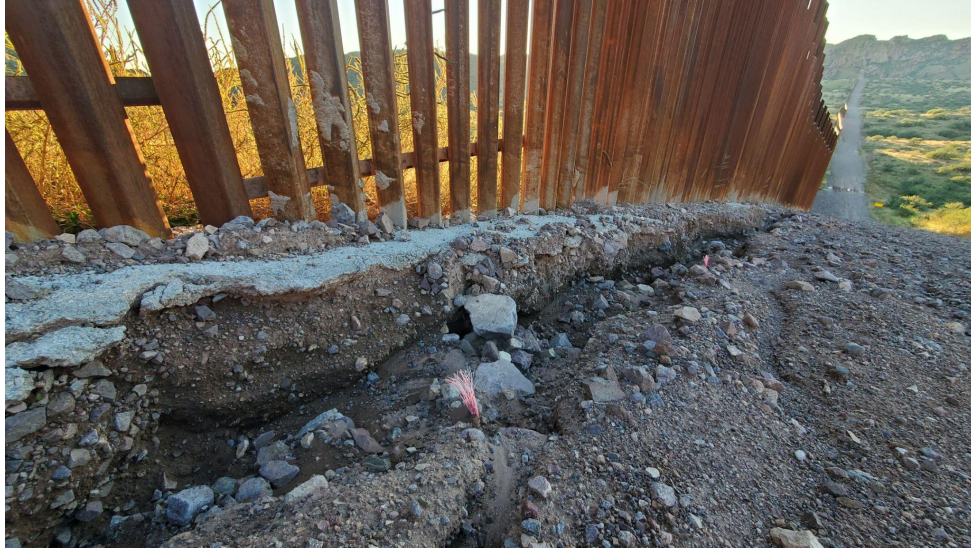
Erosion at foundation of the recently built Borderwall, photo by Erick Meza
